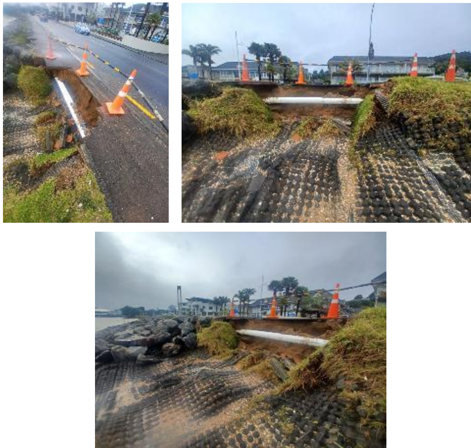
Marsden Rd Paihia footpath damage
