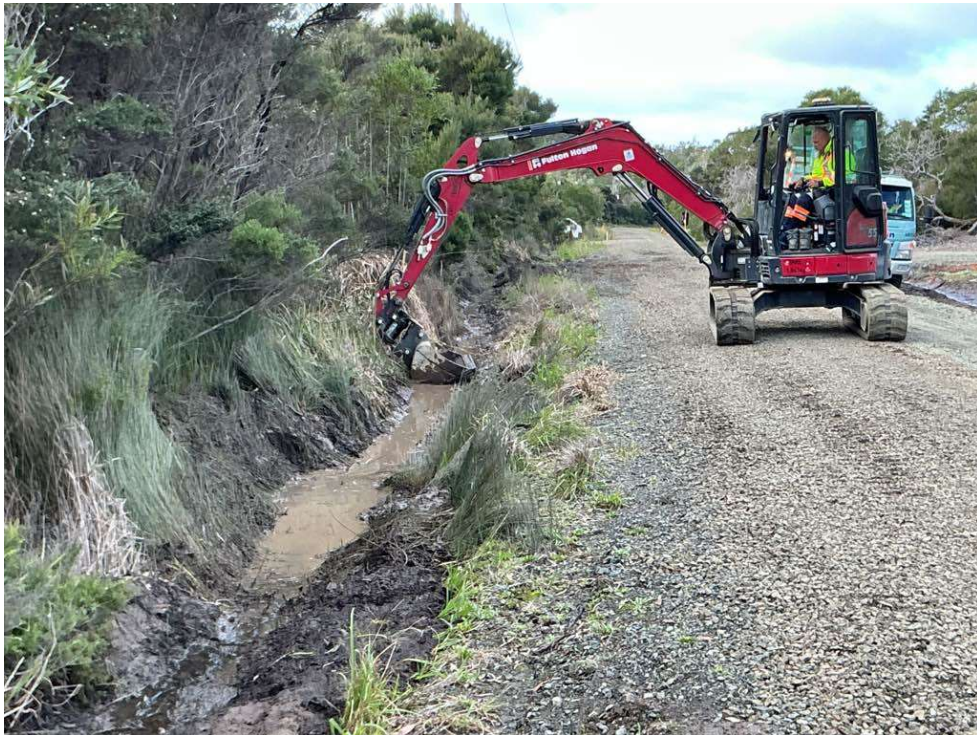
Otaipango Rd – Water tabling
