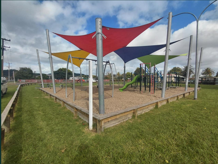
Nisbet Park Playground, Moerewa – 36m 3 New retaining wall and capping installed around playground perimeter
