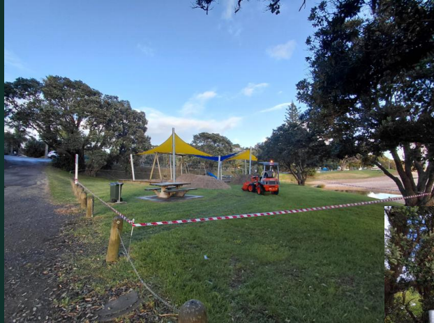
Cable Bay Reserve Playground, Cable Bay – 42m 3 New capping installed around retaining wall perimeter
