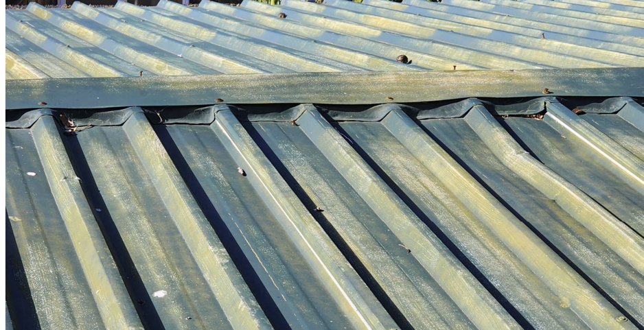
Lifting roof nails and degraded roof finish
