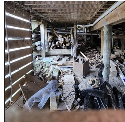
Fire risk - materials stored under building
