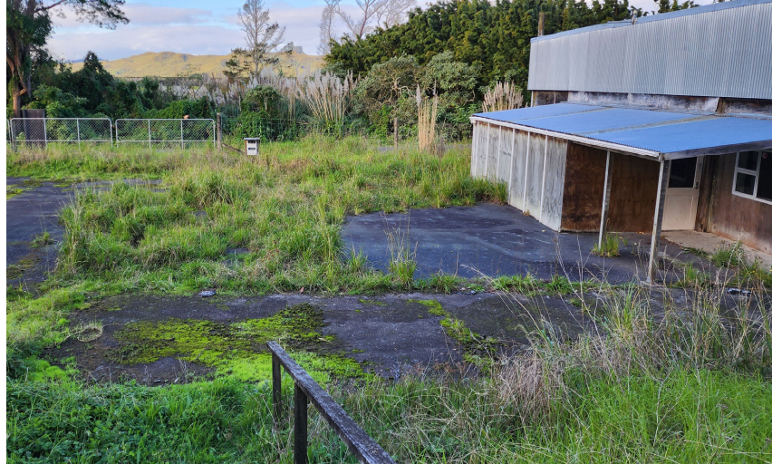
Overgrowth and damaged/non-compliant plywood claddings
