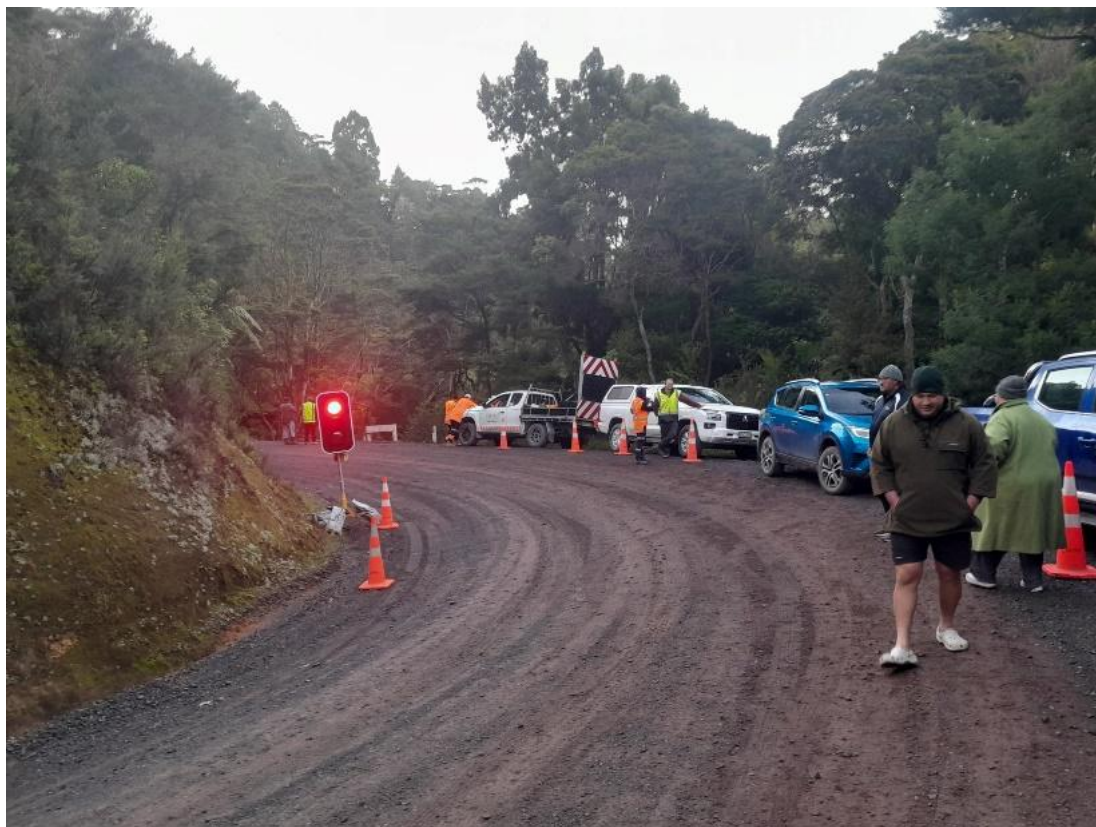
FNDC staff, contractors and local hapū whānau of Te Kapotai and Ngāti Maanu gather to offer karakia prior to the commencement of slip repairs on Waikare Road.
