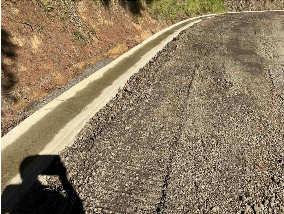
Pawarenga Rd – Storm Damage repair scour around Kerb
