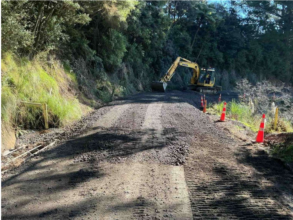
Pawarenga Rd – Storm Damage Top up underslip
