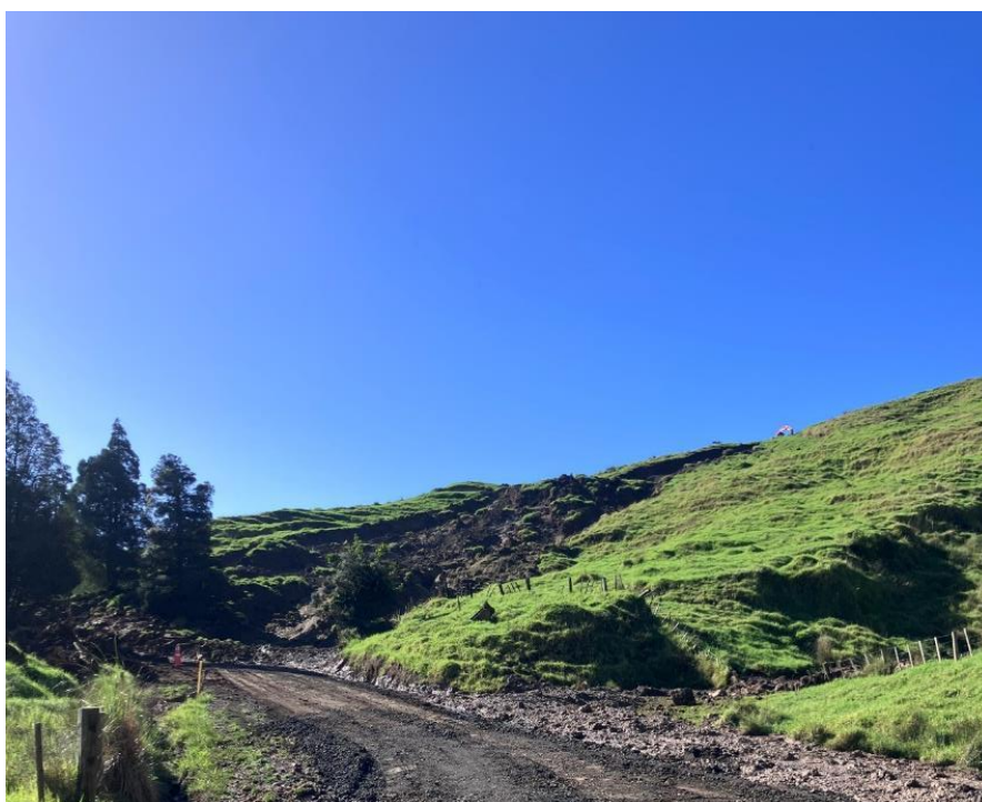
Runaruna Road Overslip
