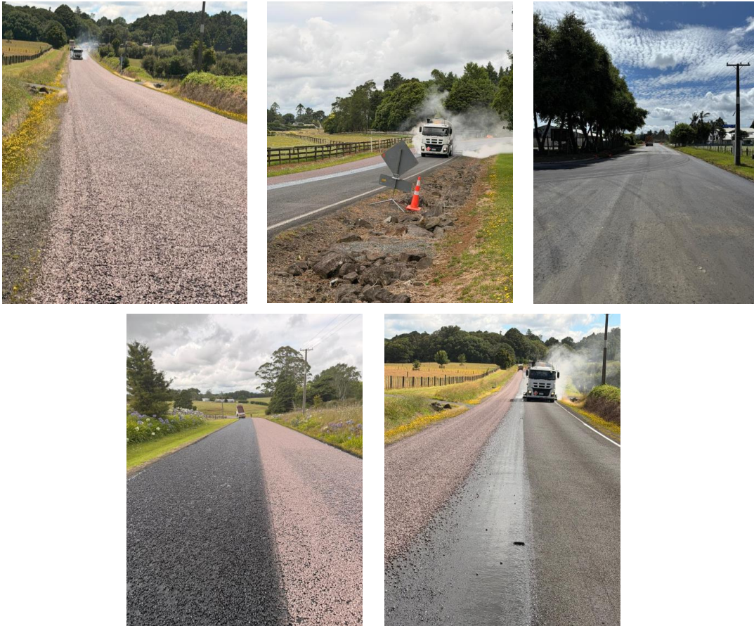
Showground Road / Carey Road AC
