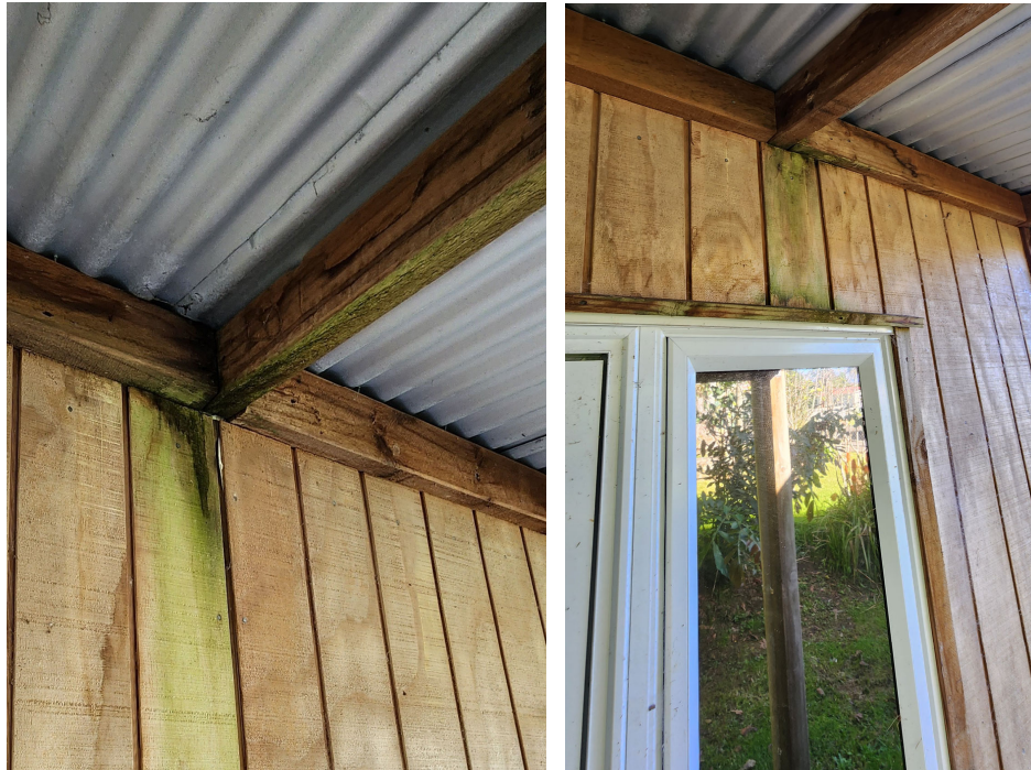
Roof leaks at wall to rear patio roof
