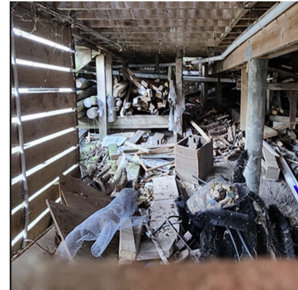
Fire risk - materials stored under building
