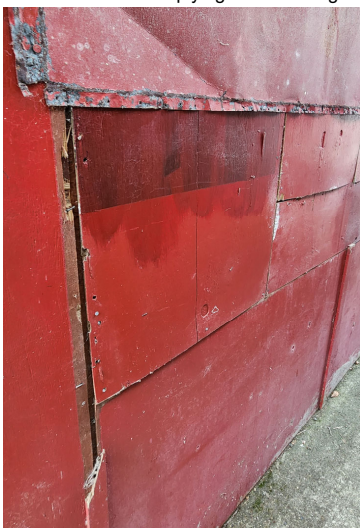
Deficient & non complying wall claddings
