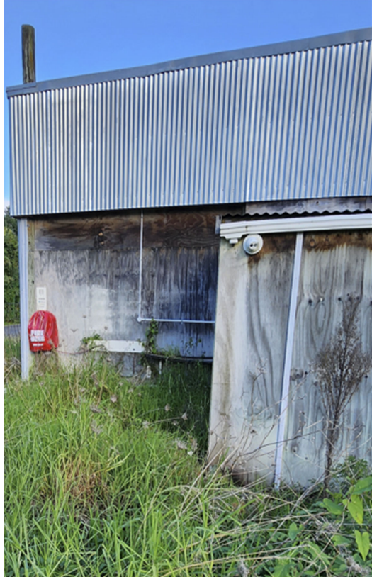
Clear vegetation away from building
