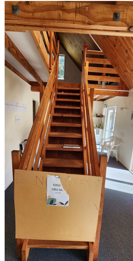
Interior mezzanine unusable due to structural/compliance deficiencies
