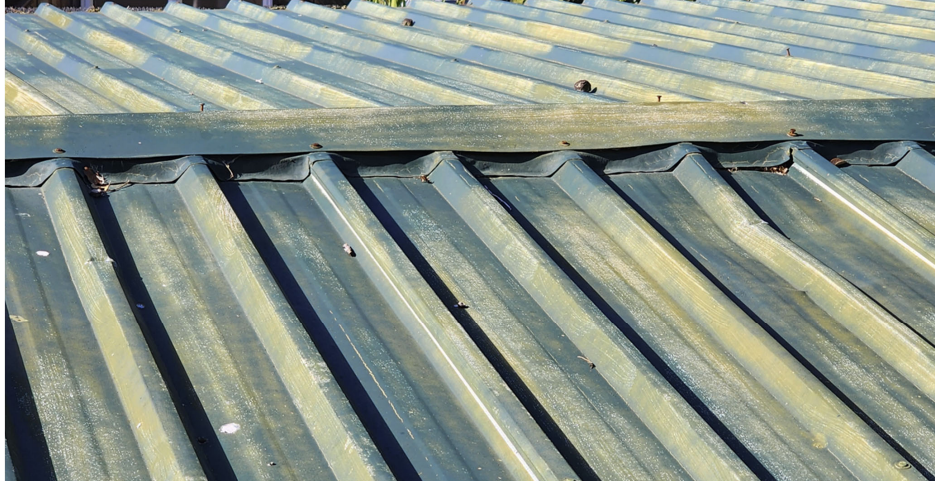
Lifting roof nails and degraded roof finish
