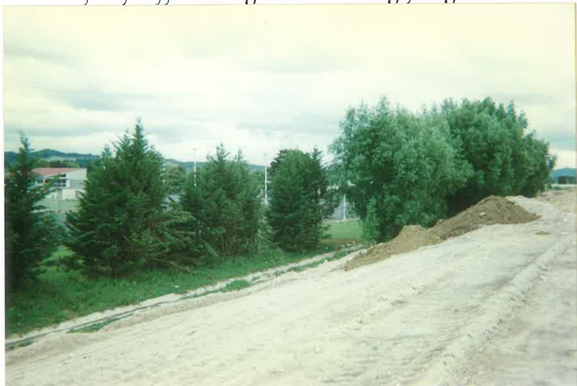
View Along Eastern Batter Slope. Willow Trees Are Being Progressively Removed As Clay Capping Proceeds
