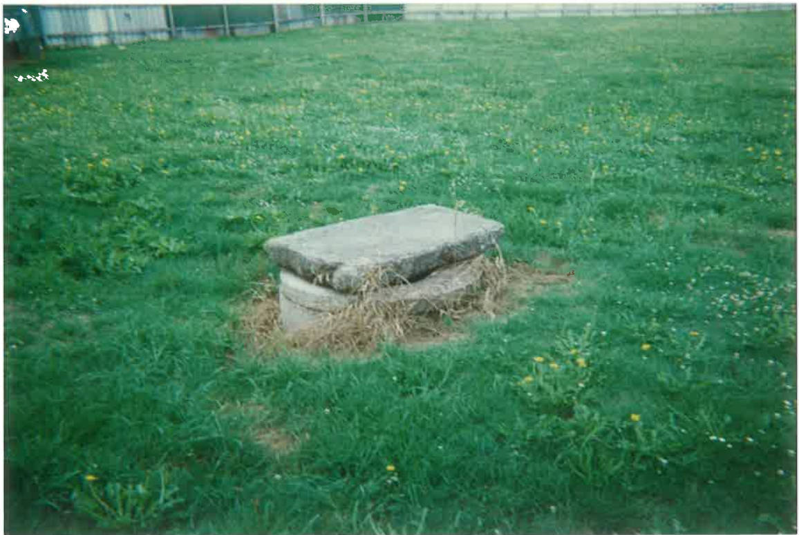
Stormwater Manhole At Eastern Side of Rugby League Field
