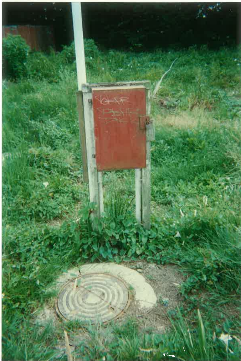
Leachate Pump Chamber With Telemetry Chamber
