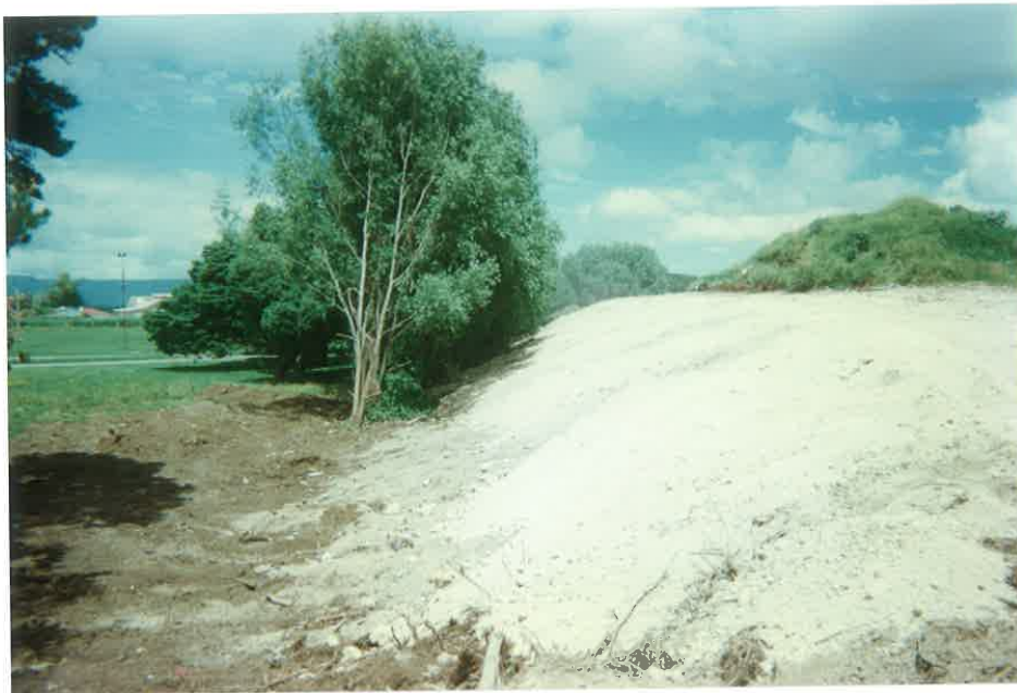
Willows Removed & Clay Capping In Progress On Southern Batter Slope (Note: Topsoil Stockpile On Landfill Crown)
