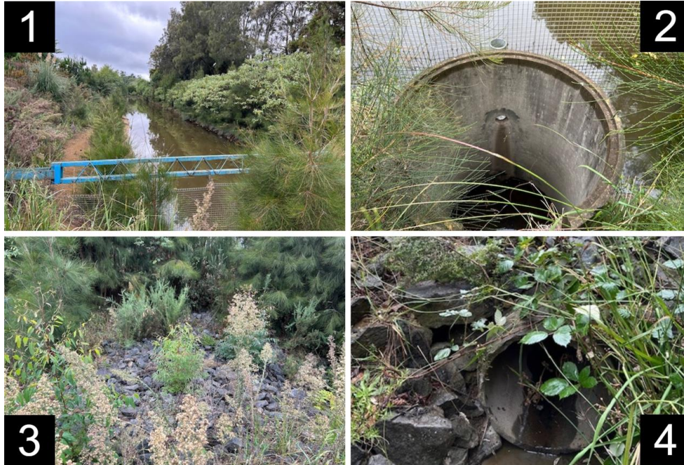
Figure 5: Photographs of the site's existing stormwater pond and culvert outlet (Source: Haigh Workman)
