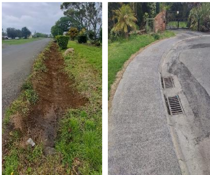
Hobson St Water tabling / Te Haumi Dr Footpath
