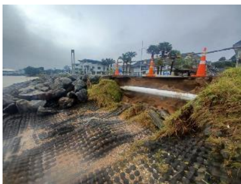
Marsden Rd Paihia footpath damage
