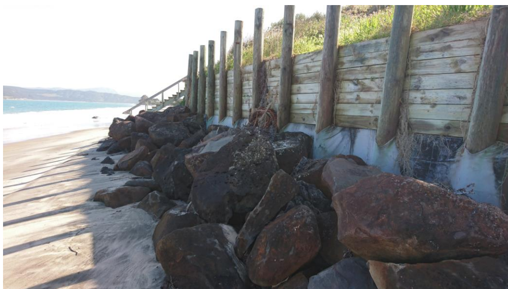
Photograph 2.4b: Combination rock rip-rap and timber armouring
