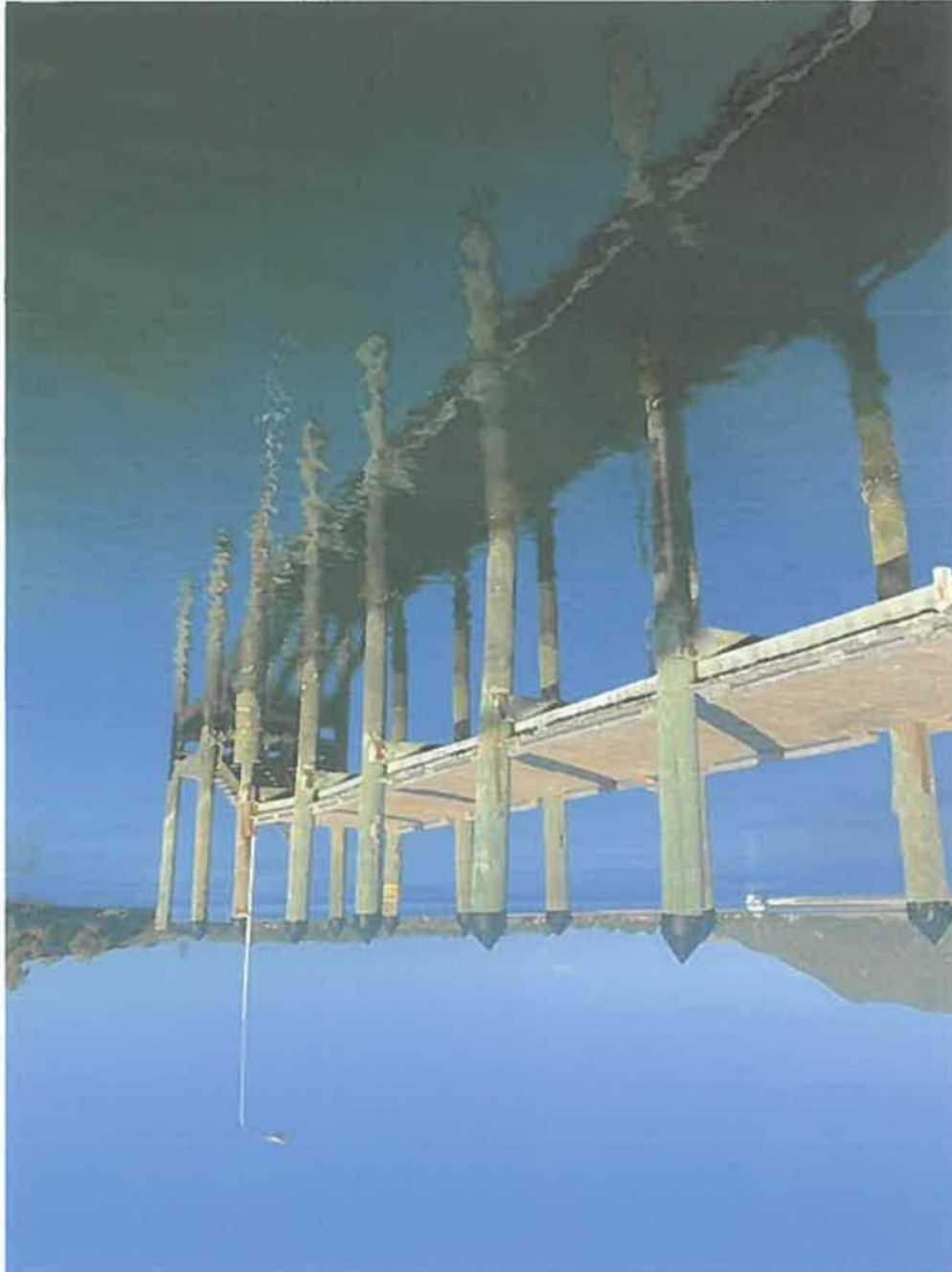
Photograph showing potential hazard of loading and unloading vessels at wharf at low tide.
